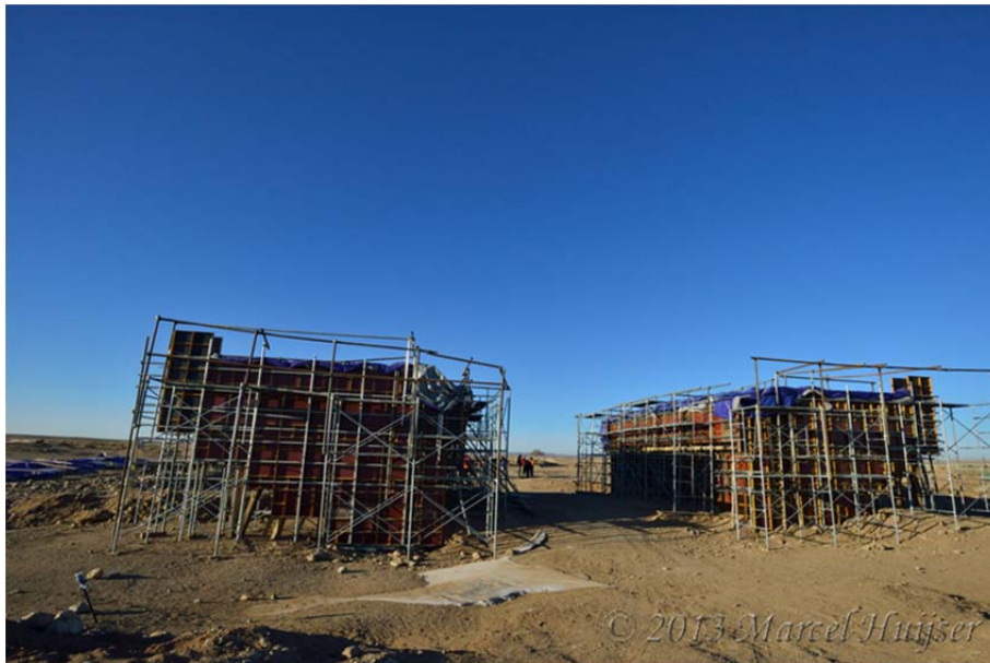
Figure 37: Bridge (about 10-12 m wide) under construction on road section from Oyu Tolgoi (mine site) to Gashuun Sukhait (border Mongolia/China), Gobi, Ömnögovi, Mongolia (© Marcel Huijser). This bridge is designed for water that may flow here after rare rain fall. The structure may also be used by wildlife under certain circumstances.
