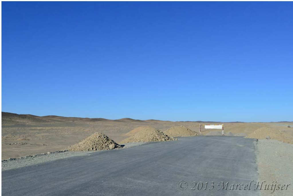
Figure 3: Finished and unfinished road section from Oyu Tolgoi mine site to Gashuun-Sukhait border crossing with China, Gobi, Ömnögovi, Mongolia (© Marcel Huijser). The paved road in the foreground is finished. Here the finished road transitions into a section that is still gravel and unfinished (background behind road closure sign).
