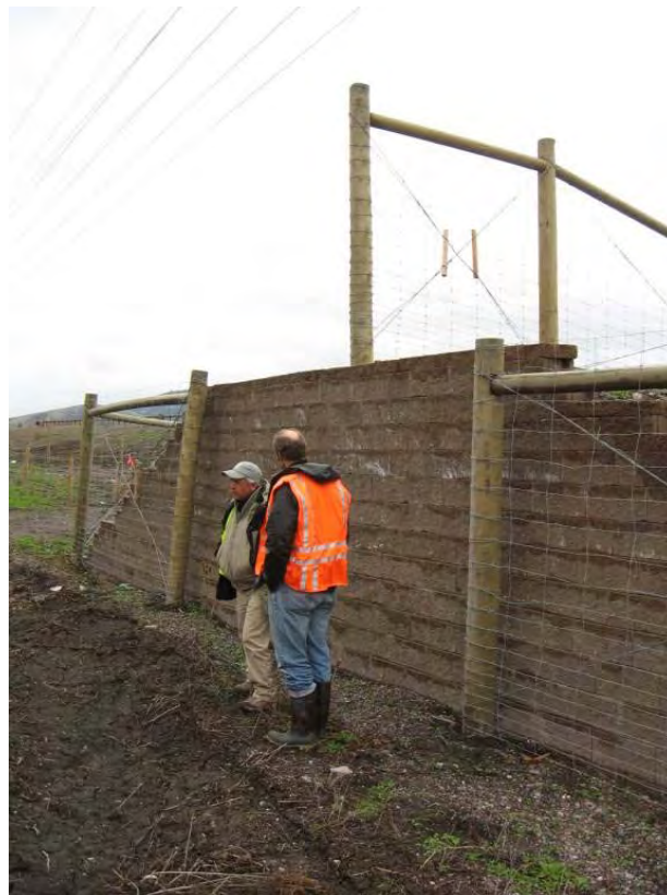
Figure 34. A jump-out along a 2.4 m (8 ft) high fence along US 93 in Montana, USA (© Marcel Huijser).
