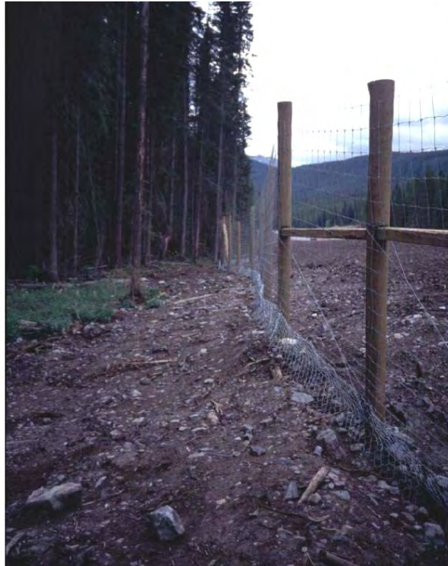
Figure 27. A 2.4 m high fence with buried apron along the Trans-Canada Highway in Banff National Park (Phase 3-A) (© Tony Clevenger).
