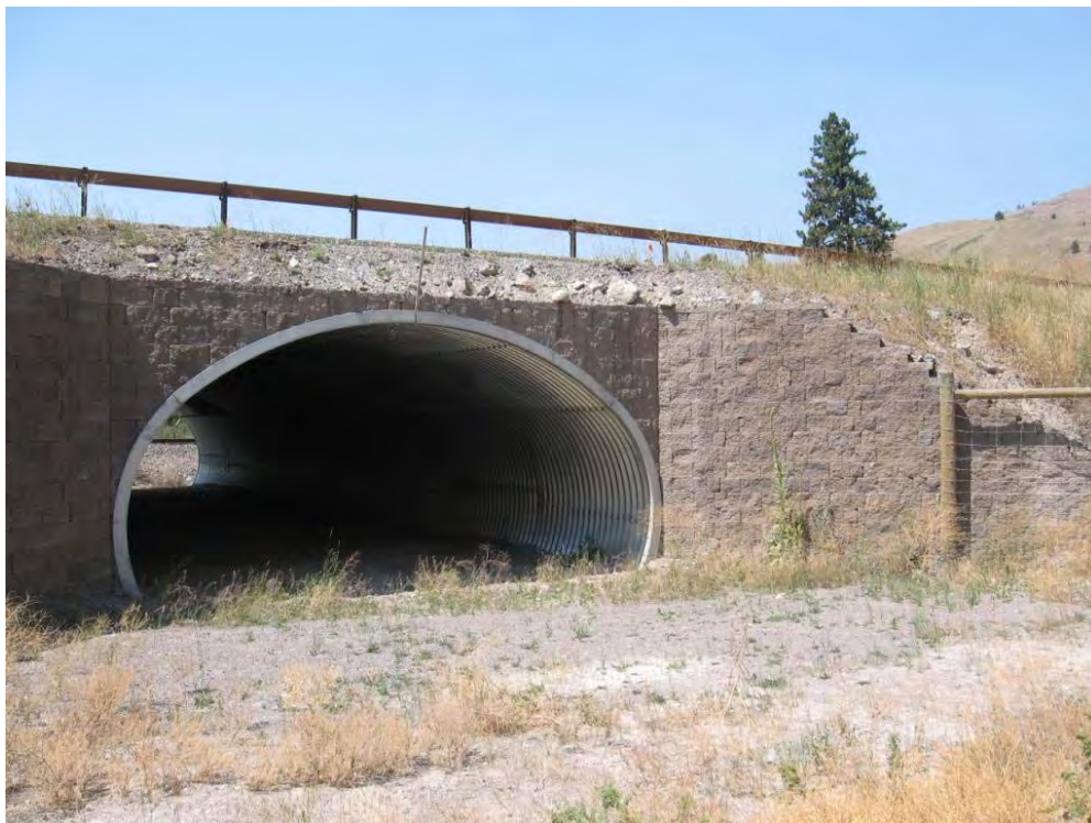
Figure 47. A large mammal underpass (7-8 m wide, 4-5 m high) along the 2-lane US Highway 93 on the Flathead Reservation in Montana, USA (south of Ravalli) (© Marcel Huijser).
