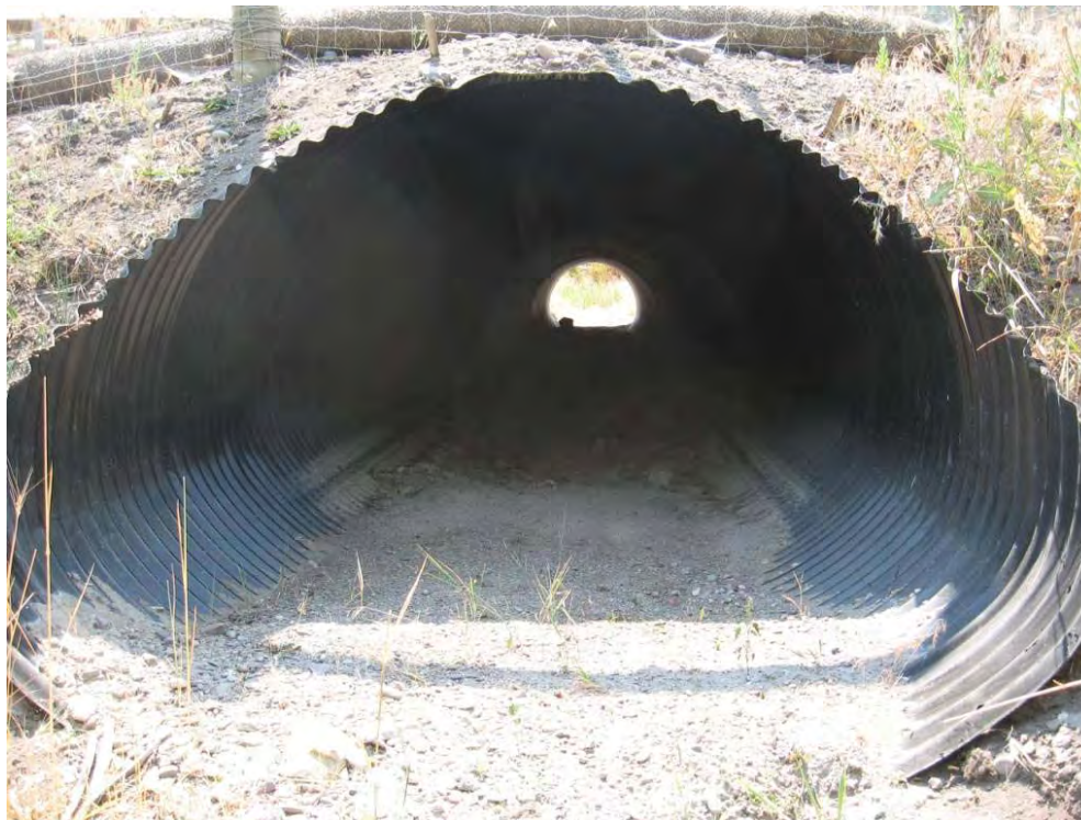
Figure 49. A medium mammal culvert (2 m wide, 1.5 m high) along the 2-lane US Highway 93 on the Flathead Reservation in Montana, USA (south of Ravalli) (© Marcel Huijser).
