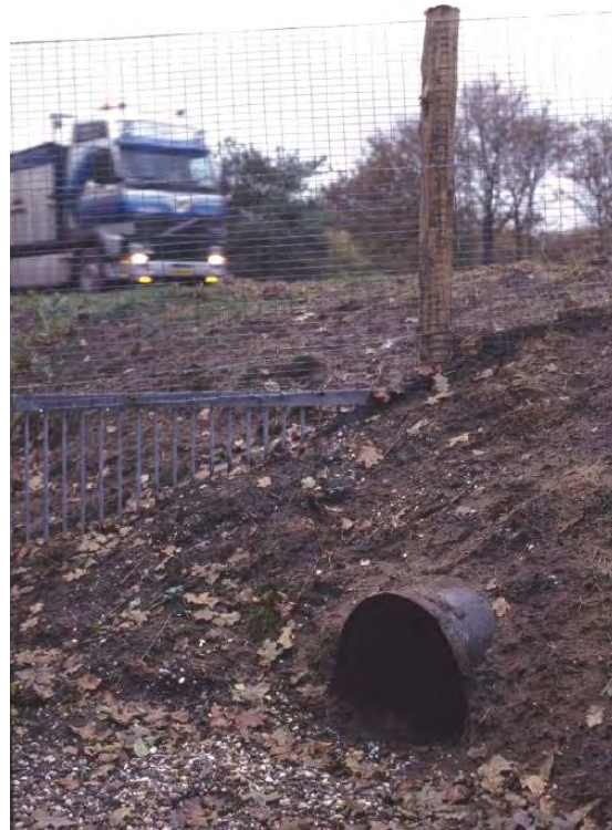
Figure 50. A small-medium mammal pipe (“badger pipe”) in The Netherlands (© Marcel Huijser).
