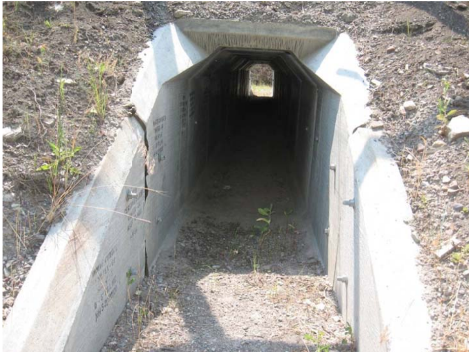
Figure 26. A medium mammal box culvert (1.2 m wide, 1.8 m high) along the 2-lane US Highway 93 on the Flathead Reservation in Montana, USA (south of Ravalli) (© Marcel Huijser).
