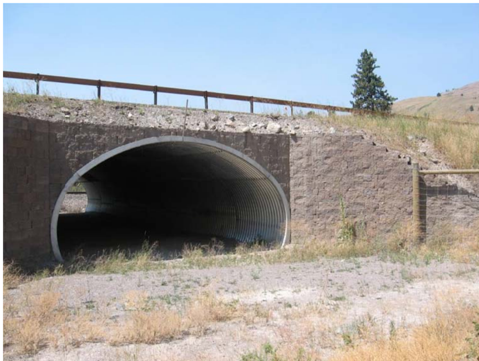
Figure 25. A large mammal underpass (7-8 m wide, 4-5 m high) along the 2-lane US Highway 93 on the Flathead Reservation in Montana, USA (south of Ravalli) (© Marcel Huijser).
