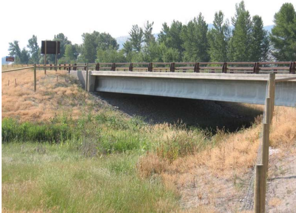
Figure 24. An open span bridge along the 2-lane US Highway 93 on the Flathead Reservation in Montana, USA (across Spring Creek, south of Ravalli) (© Marcel Huijser).
