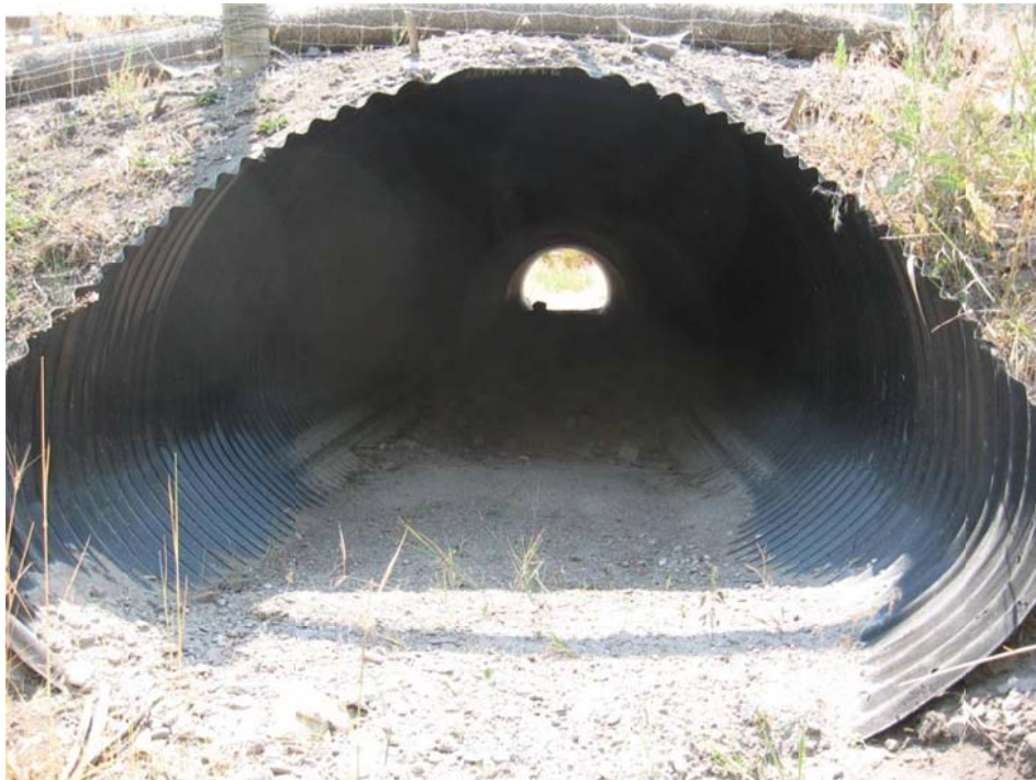
Figure 27. A medium mammal culvert (2 m wide, 1.5 m high) along the 2-lane US Highway 93 on the Flathead Reservation in Montana, USA (south of Ravalli) (© Marcel Huijser).
