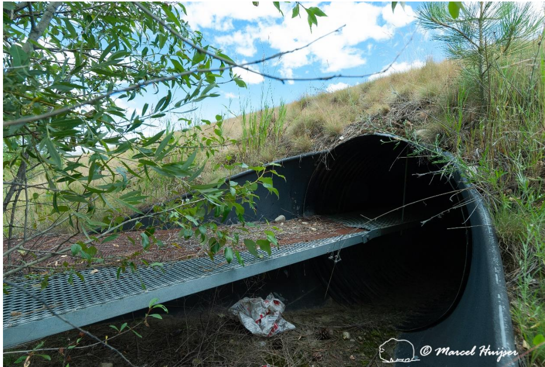
Figure 4: Metal shelving installed in drainage culvert in Montana.
