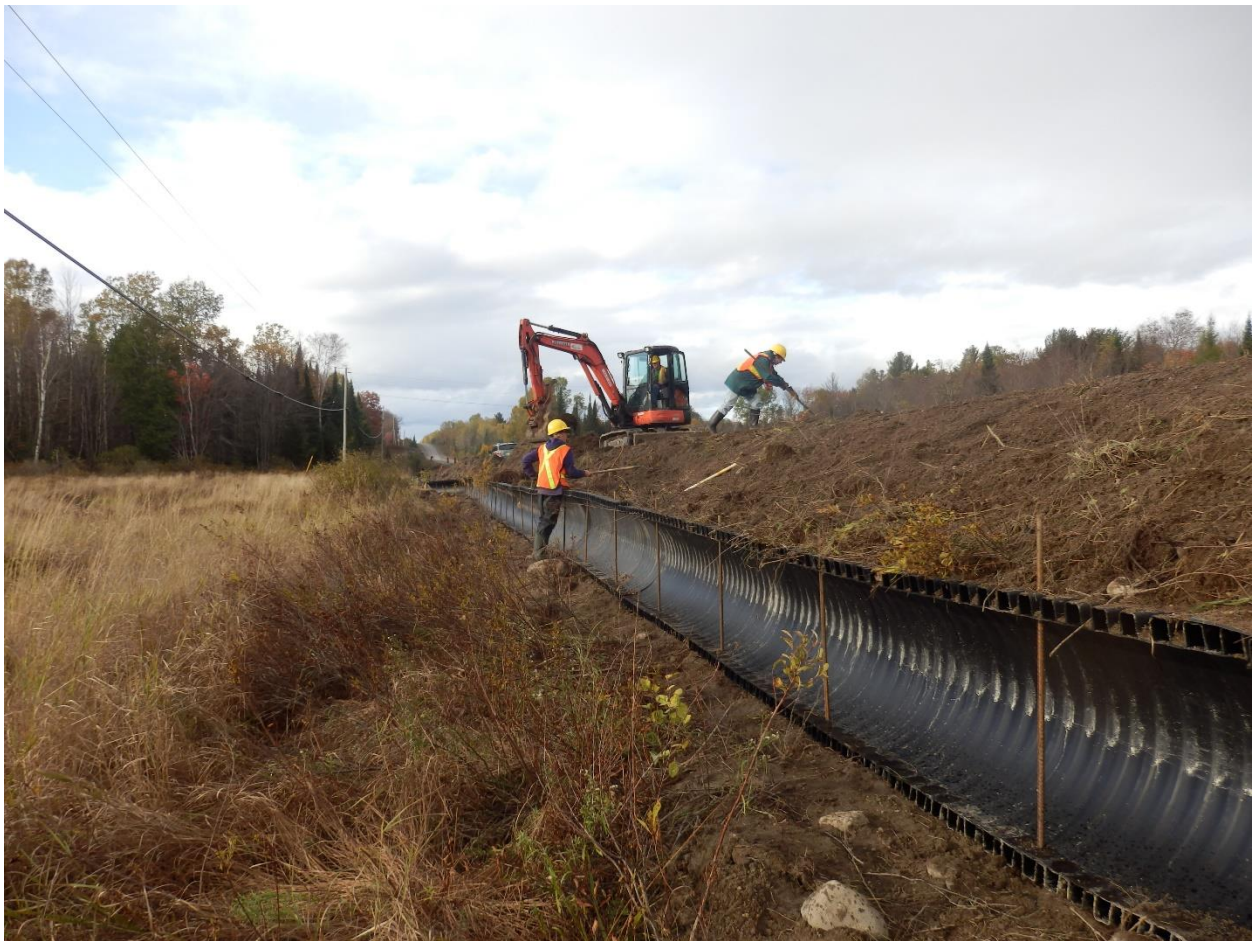
Figure 6: Boss HDPE materials used for barrier wall with back-fill and supported with steel rods. Photo Credit: Paul Heaven.
