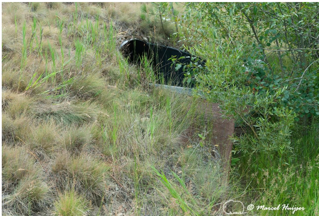
Figure 5: Ramp extending at right angle from metal shelving installed in a drainage culvert in Montana.
